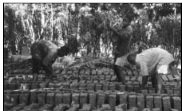
Bricks already built for the library; note worker on right wearing IU T-shirt.
