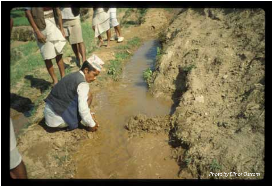
◀ Farmers repairing an earthen irrigation canal in the Dang Valley region of Nepal. Upon discovering that a local farmer had diverted the irrigation canal, the farmers immediately rushed to repair the canal and sanction the offending party.
